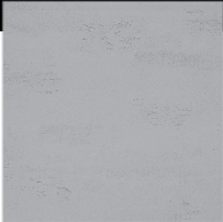
MOA-##-S | Pitted Surface
